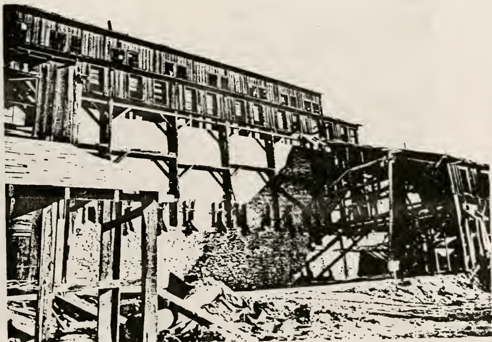
Figure 171. Arsenic plant (structure #59) showing discharge gates for emptying the primary kitchen, east view.
